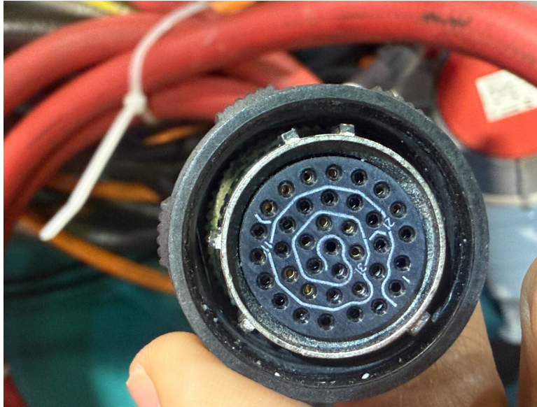
FIGURE 8: PCS-01. The pin face of the refrigeration-permit connector on the telescope-side cabling. An unseated pin here is what produced the spurious chiller trips — no chiller anomaly, a permit signal that came and went as the TMA moved. The pins and the shell were renewed (2025-04-11, #cam-operator).
